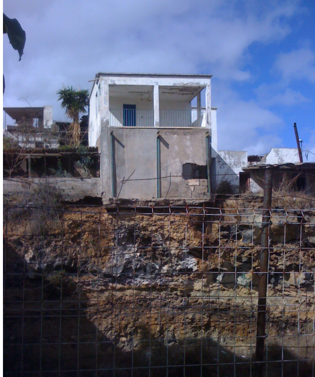
Figure 10. Photography of a house in Tenerife. The poor foundations and the different volcanic strata underneath can be seen
