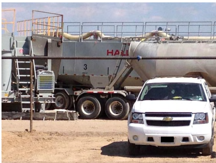
Figure 2: Large Tanks (in background) are pumping the water/sand mixture into the ground. Note water truck supplying water for operation (in foreground).
