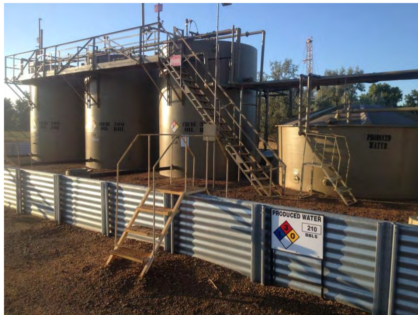
Figure 5: A 400-gallon tank battery in which oil is stored. The smaller tank holds the separated water. The separated gas has already been sent through the pipeline.
