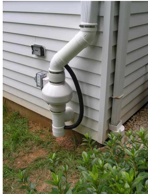
Photo 4 - System with Dilts by pass drain
