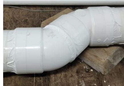
Figure (30): Six inch angled 45 degree offset pipe fittings
