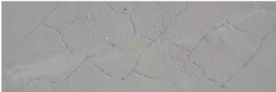
Figure (9): Cracks in single application of epoxy
