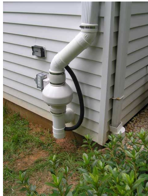
Photo 4 - System with Dilts by pass drain
