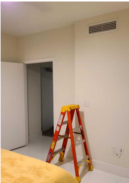
Figure (26): Bedroom/office return grill
