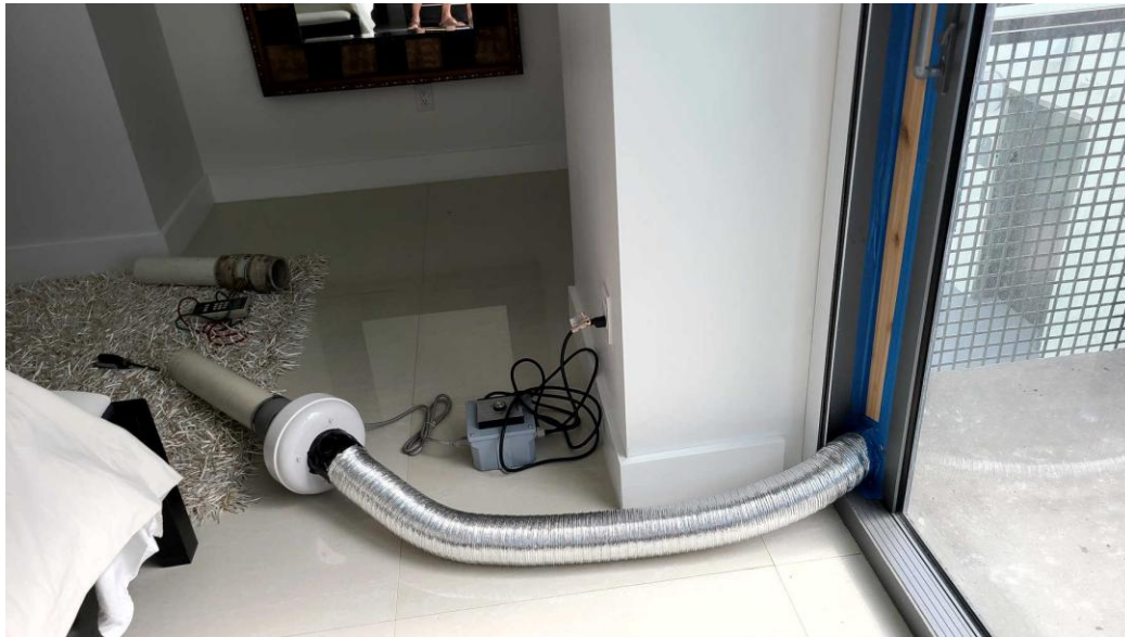
Figure (14): Ventilation equipment and flow grid equipment
