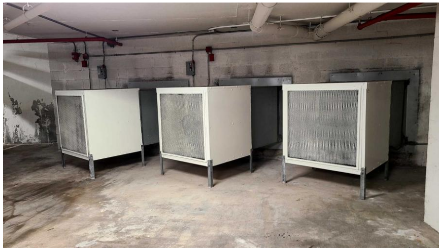
Figure (6): Garage exhaust fans
