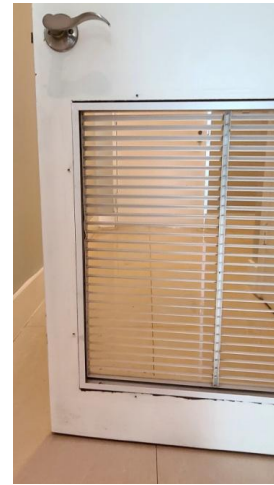
Figure (21): Non restricting return grill
