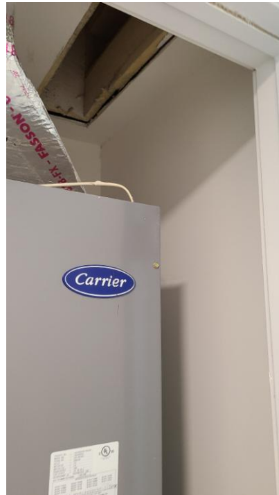
Figure (25): 4X6 duct installed in wall of HVAC closet with adjustable grill
