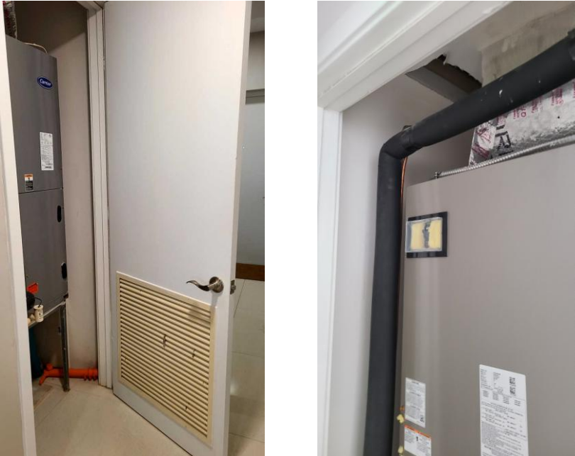
Figure (18) HVAC closet with limited space and return grill.
