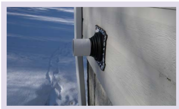
Photo 10 - Example of a ground level exhaust discharge
