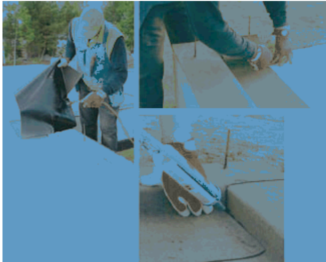
Figure 5 Handling of bitumen felt and seaming of the strips in the corner.
