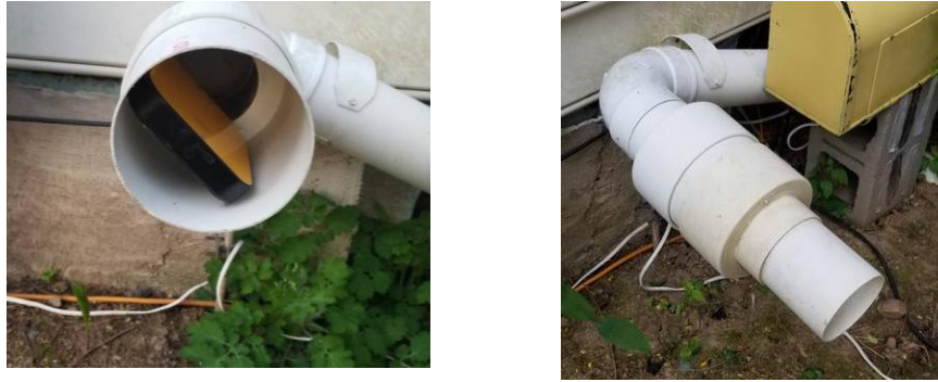
Figure 8 - Corentium Pro installed in exhaust piping
